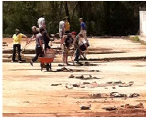
The youth are faithfully working on the second Hampton Avenue parking area.
